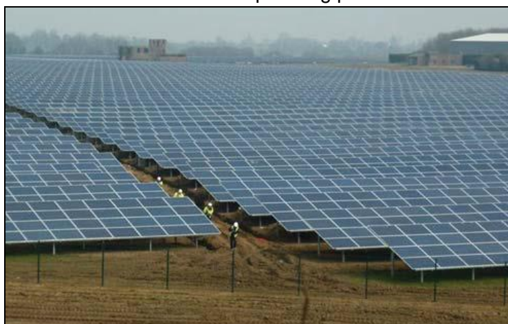
The solar photovoltaic farm at Wymeswold Airfield
